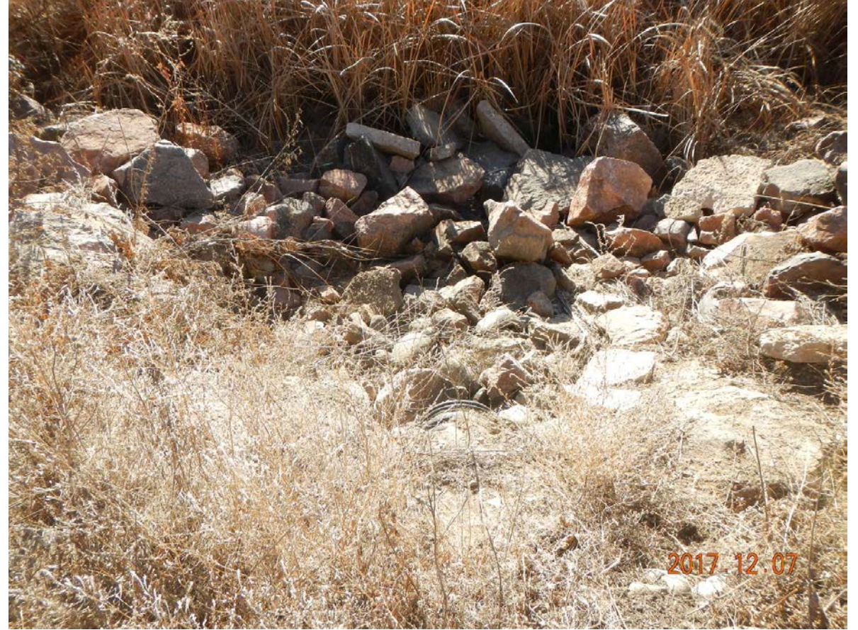
14_Seepage, previous failure
