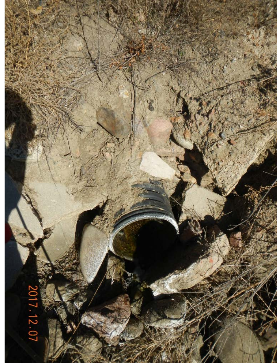
12_Seepage, previous failure
