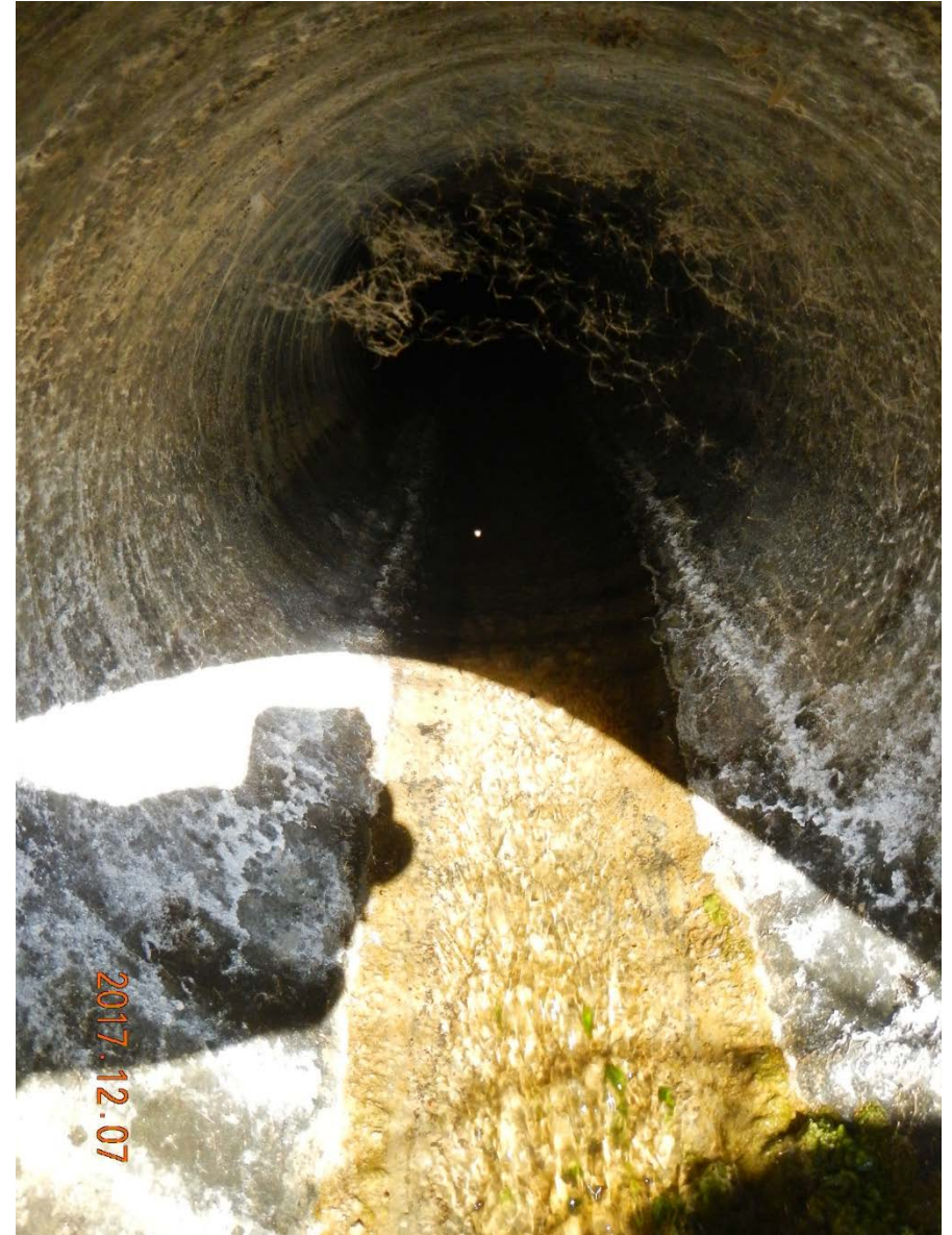
15_Seepage, previous failure
