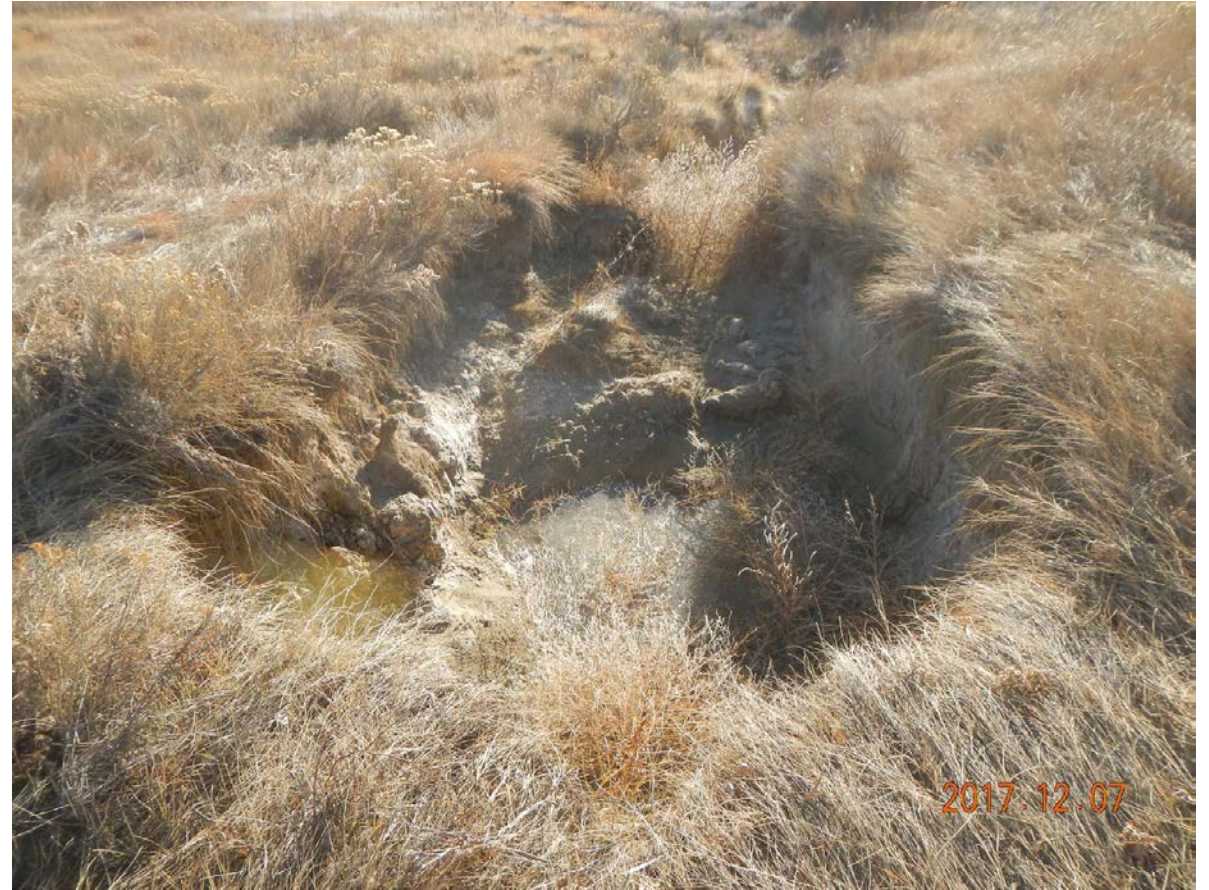
24_Em Spwy headcutting
