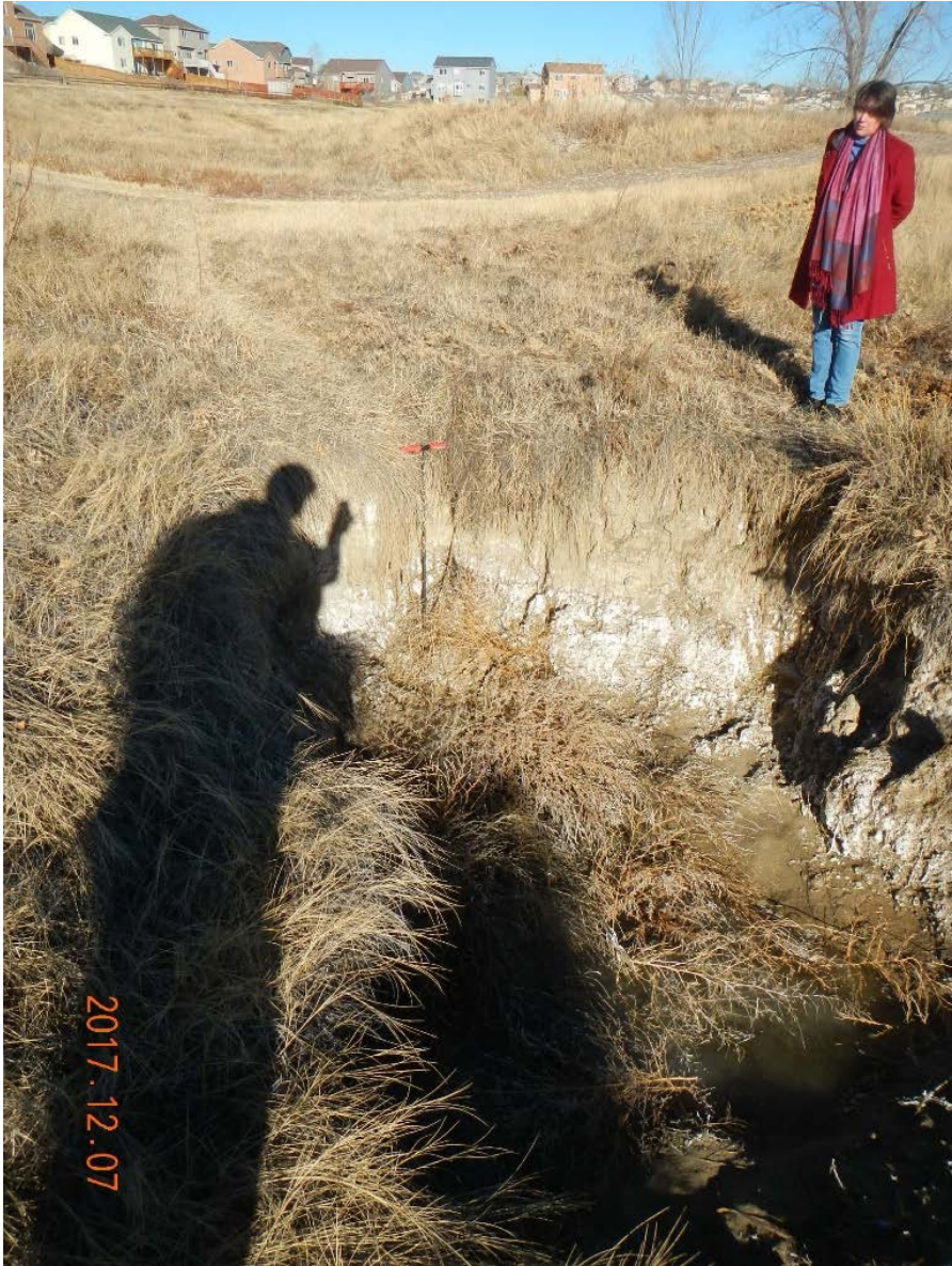
25_Em Spwy Headcutting
