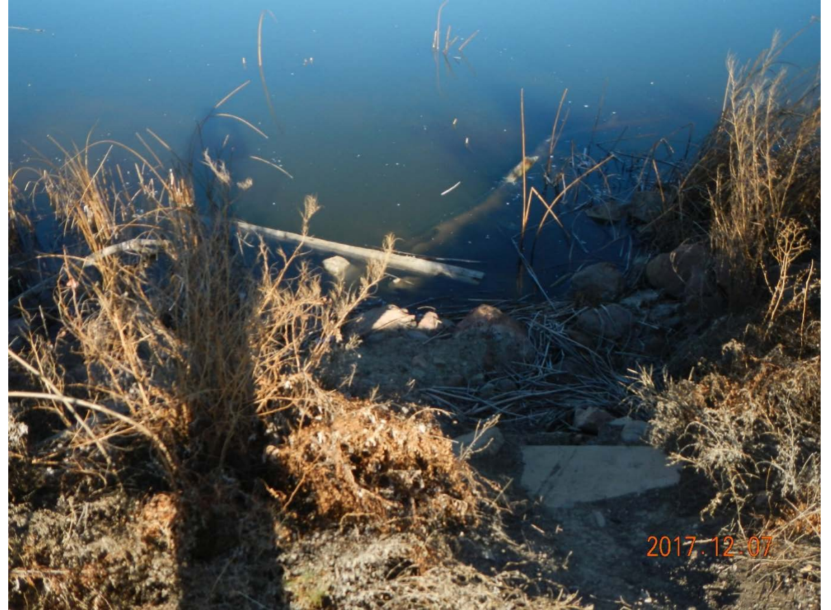
04_Upstream Slope, previous failure
