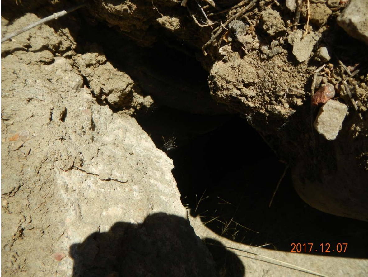
13_Seepage, previous failure
