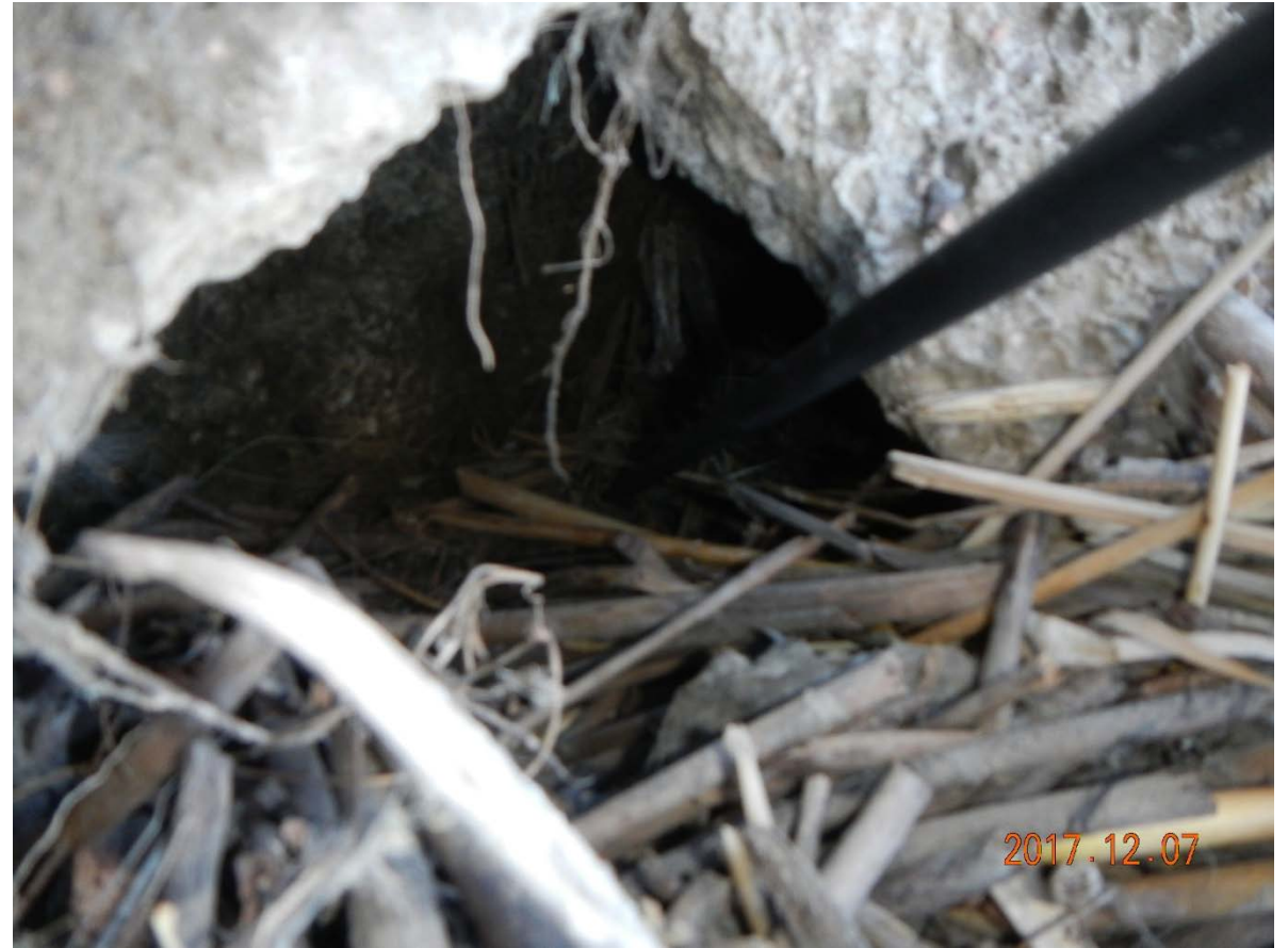
06_Upstream Slope, previous failure location
