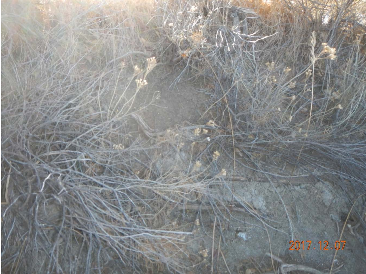
03_Upstream Slope, roots
