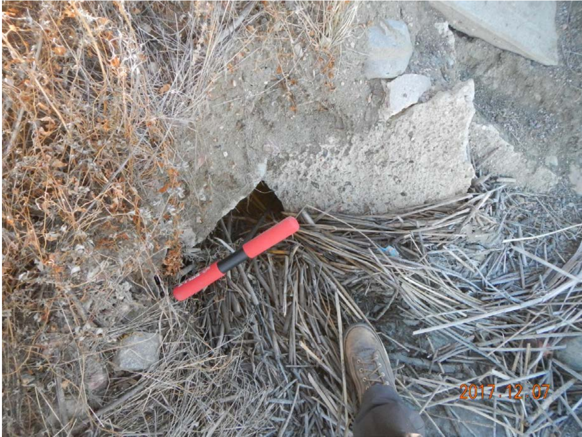
05_Upstream Slope, previous failure location
